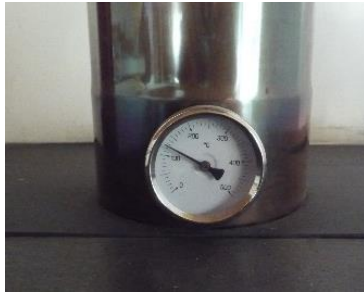
The exhaust gas temperature drops Down to about 130 – 160 °C
